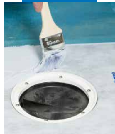
Butyl gasket (self-adhesive end) is laid over the drain (on primed floor). Then apply Mapegum WPS over the gasket and the rest of the floor
